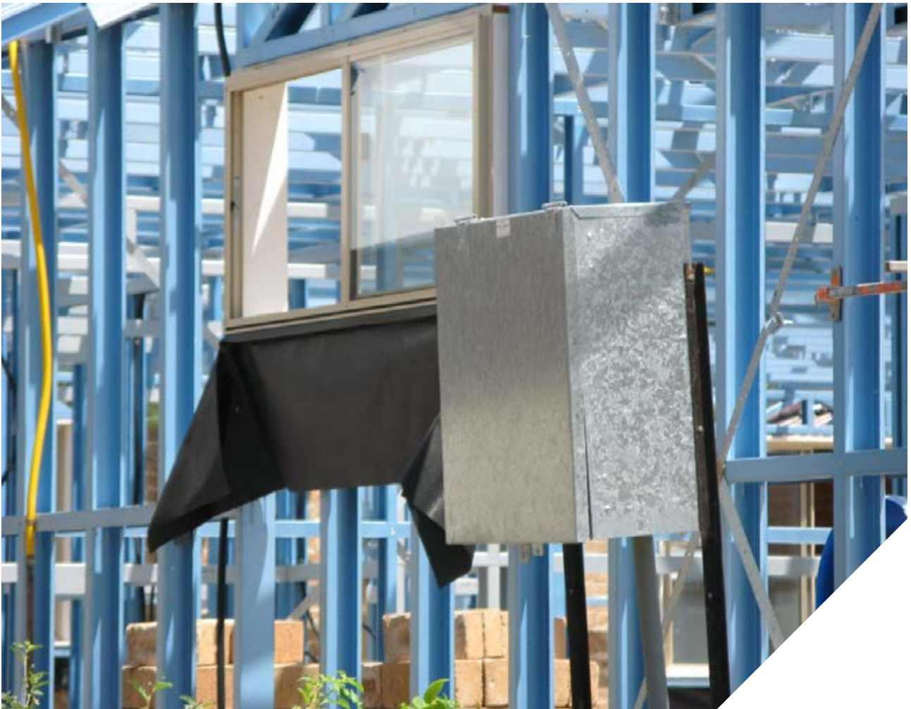
Temporary meter box
