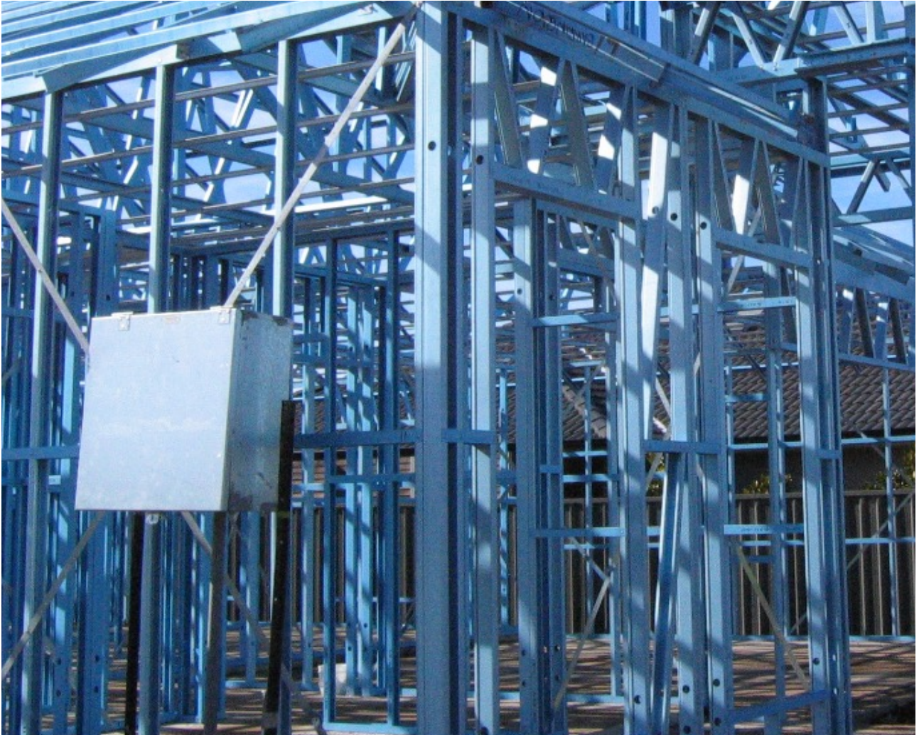
Temporary meter box
